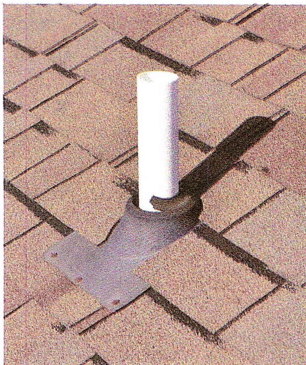
Failed temporary pipe boot causing leaks and water damage
